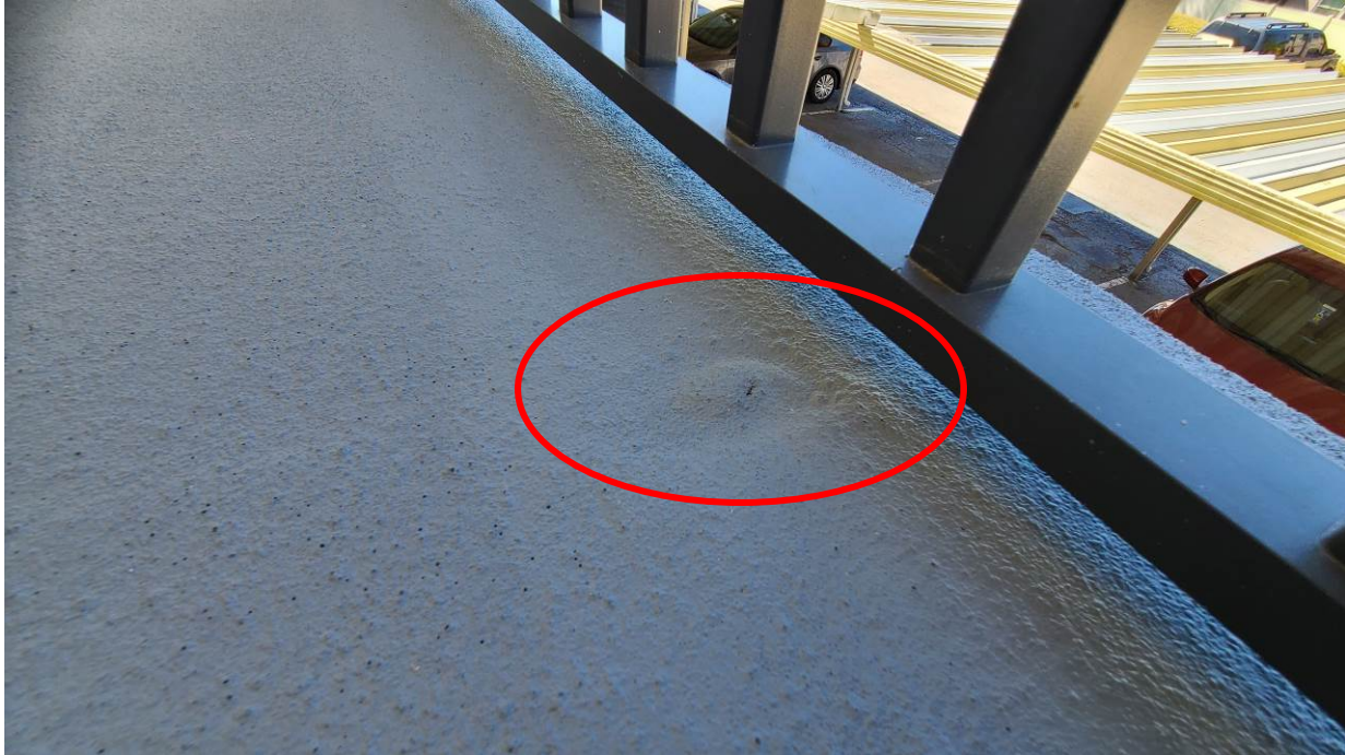
Photograph 13: Blistered Deck Coating near Elevator Door on 2 nd Level Walkway
