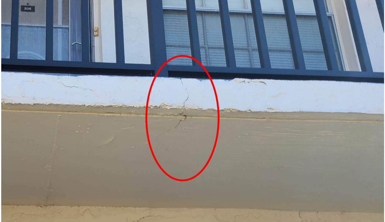
Photograph 15: Spalled Walkway Edge near Unit #206
