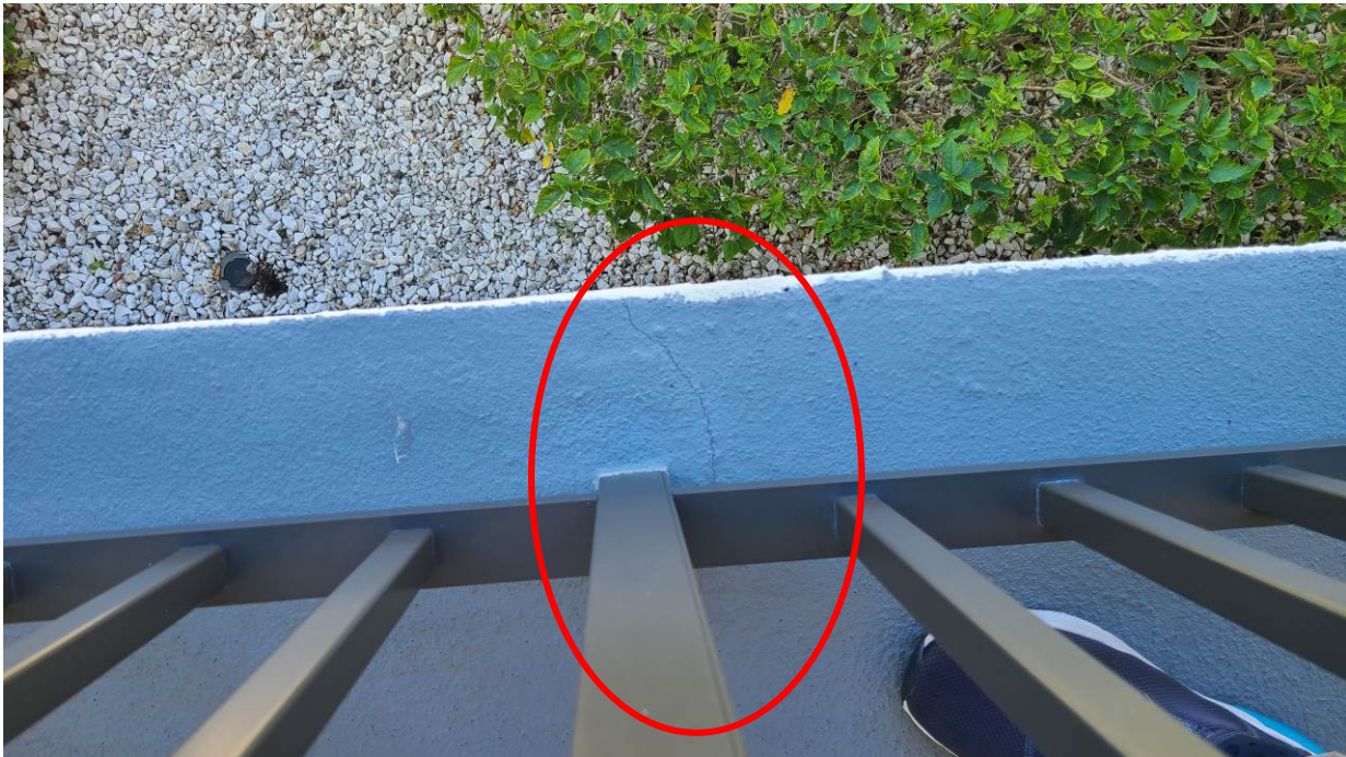
Photograph 14: Cracked Deck Coating near Unit 206
