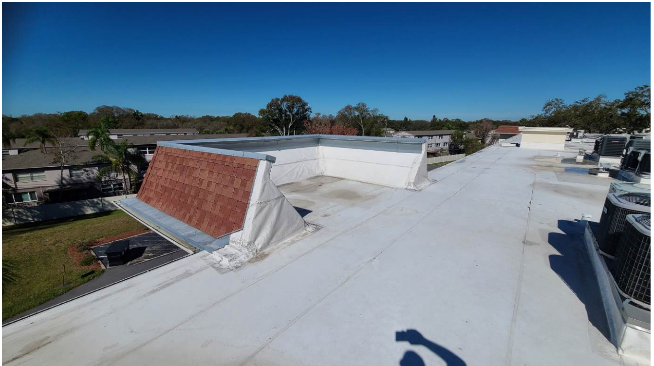
Photograph 5: Close Photo to Building the Flat Roof and Mansard Roof – Reported was Installed around May 2004
