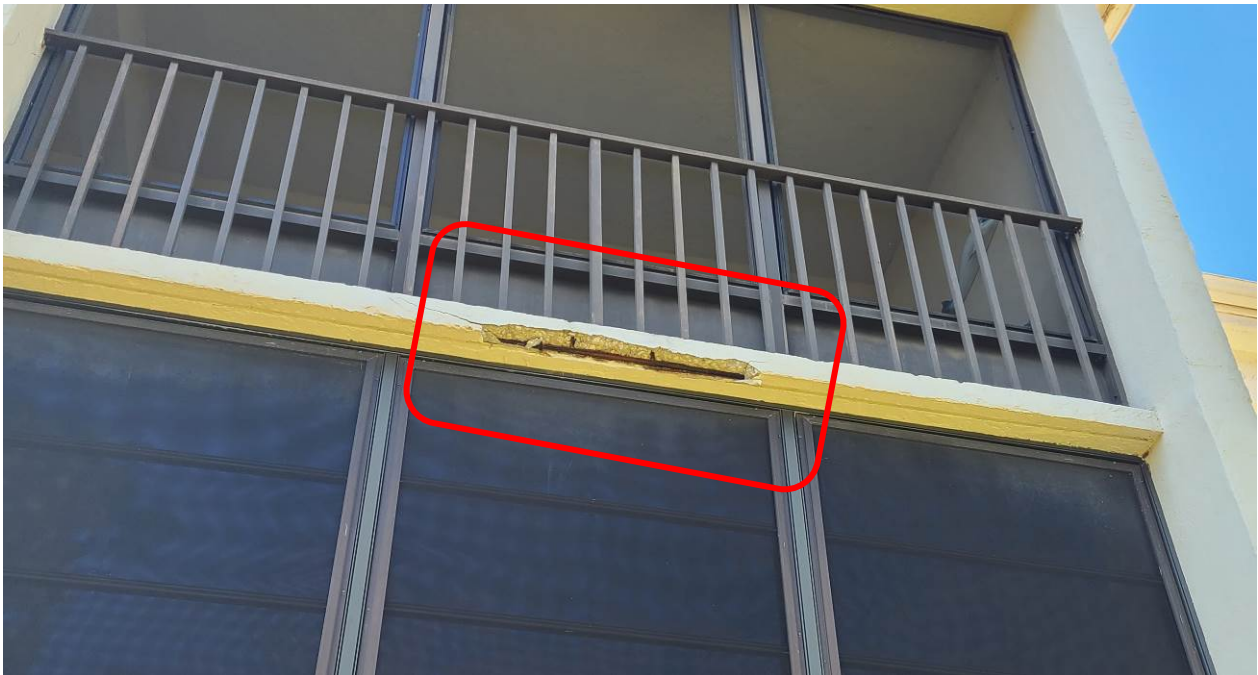
Photograph 16: Spalled Balcony Edge at Unit #308
